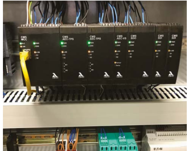
CMS modules installed in the control cabinet.
